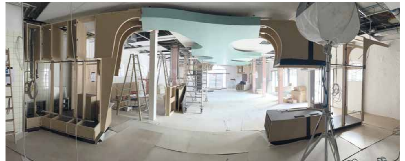
Master craftsmanship: Schirm installs the ceiling construction of the “Kraken” at the end of March
