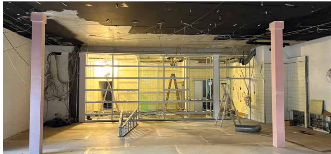
This is how it looked at the beginning of February 2023. The shelves for the breeding room are already in place in the background. But before things can get started, all the water pipes, ventilation and electrics have to be installed on the ceiling.
