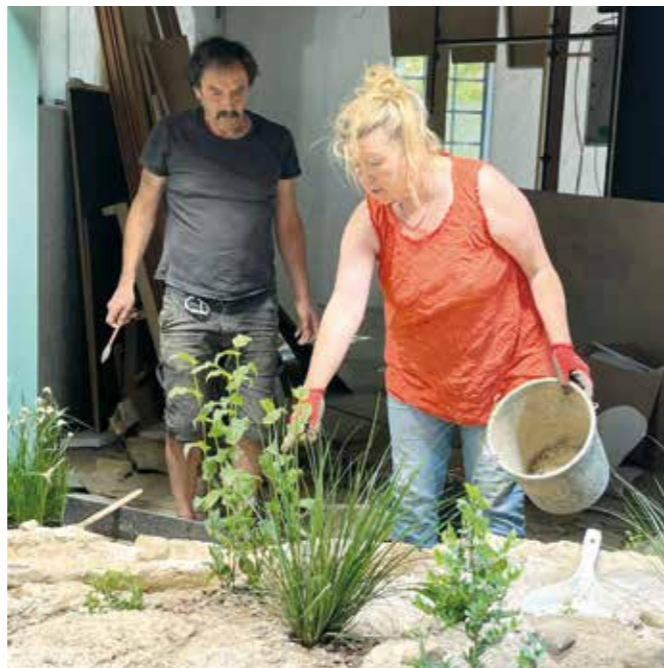
Construction site ping-pong. While Sabine Hohmann starts planting the toad enclosure, Oliver Blomeier is still optimising the watercourse.
