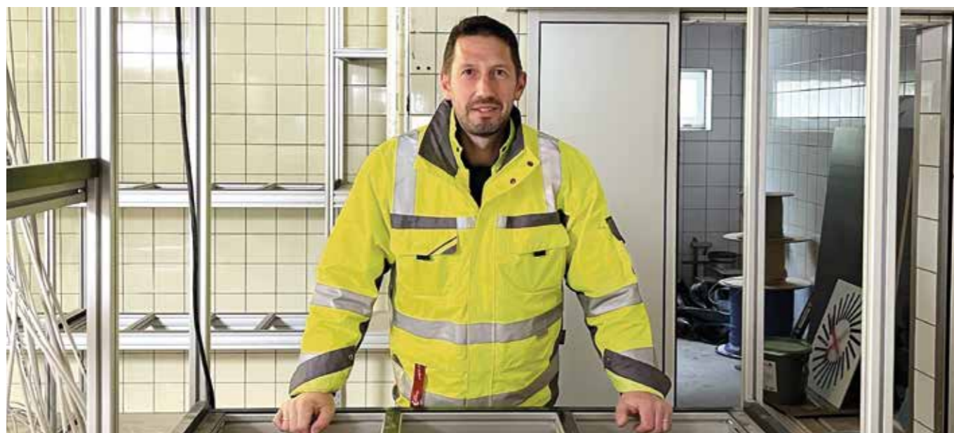
You need a calm mind – zoo site manager Marco Hustedt has the wonderful task of orchestrating all the trades on the construction site.
