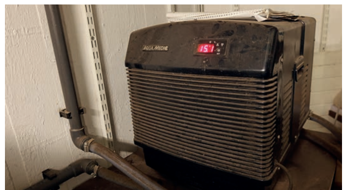
Cooling unit for setting the required low water temperature | Sebastian Rohling
