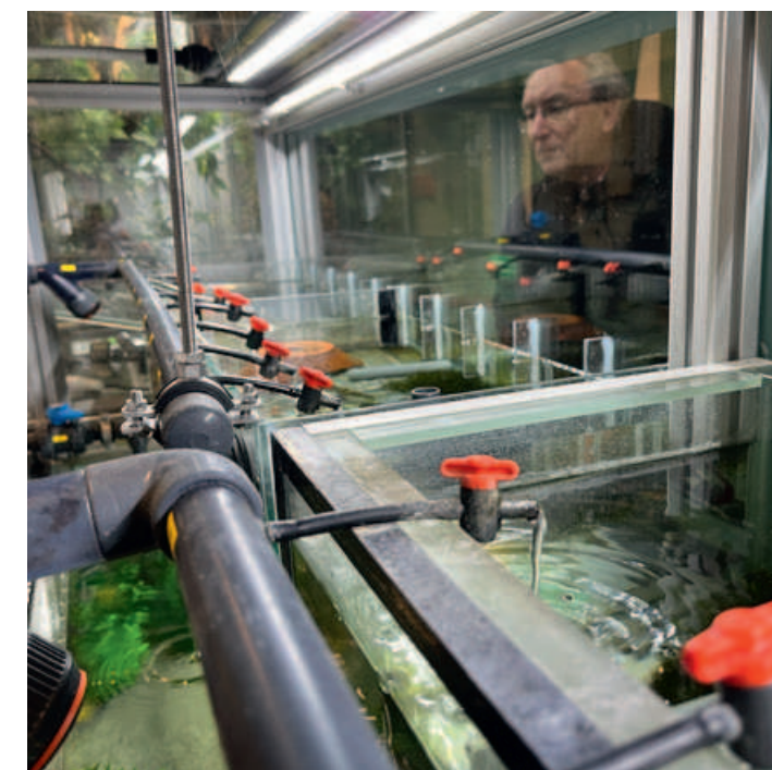
In contrast to the habitat sections in the exhibition, the technology here is deliberately made clearly visible.
